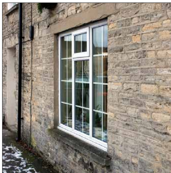
Fig. 7 An inappropriate modern uPVC double-glazed window
