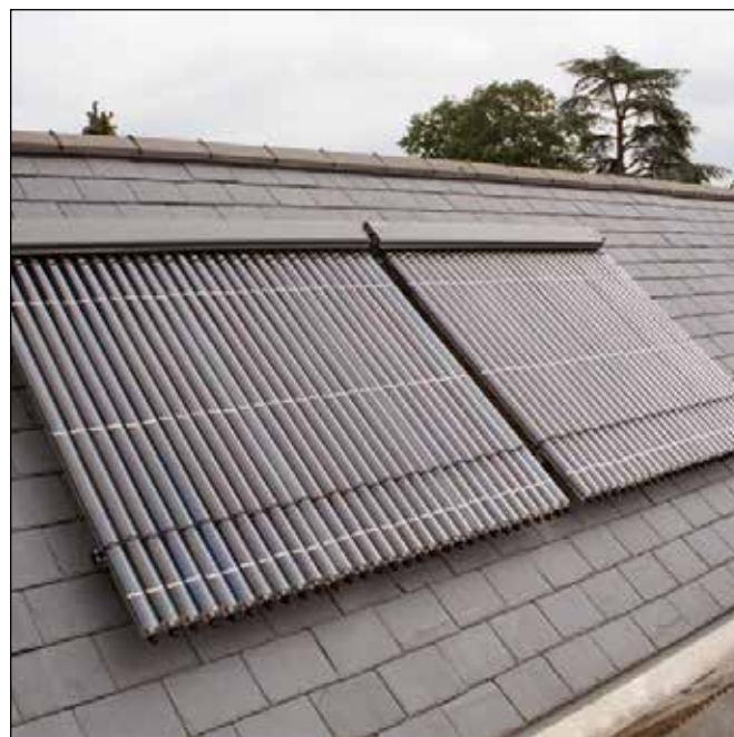
Fig. 14 Solar thermal panels (evacuated tube type)
